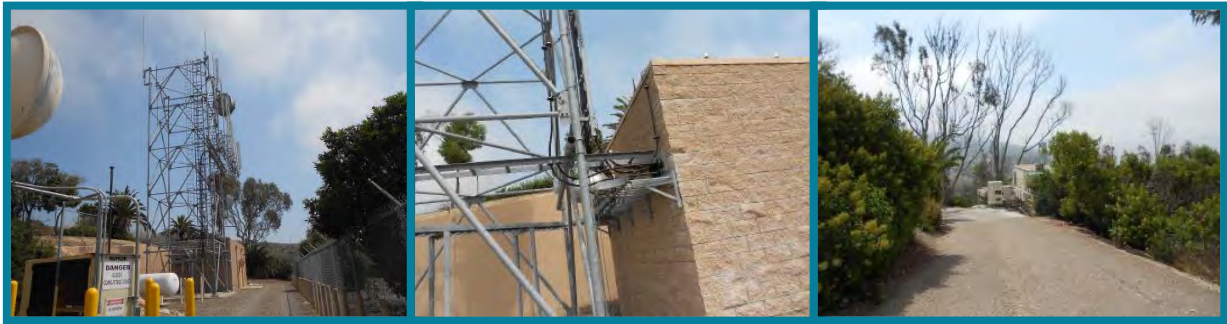
Antenna Tower at Moorhead Reservoir
