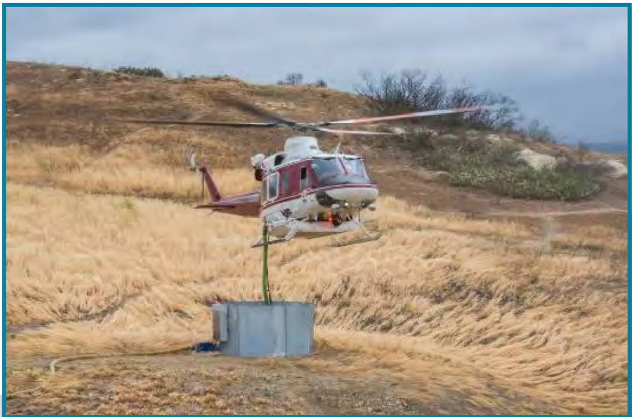
Helicopter refilling its tanks from a RASS fire hydrant without assistance
