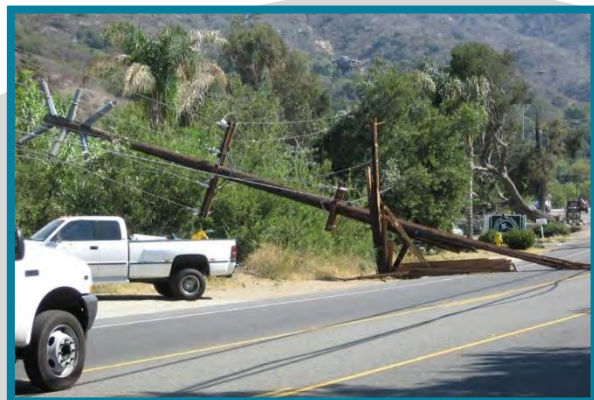
2007 Pole Down on Laguna Canyon Road
