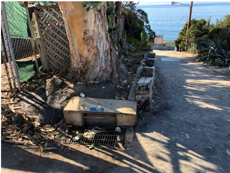
Photo 2: View of the inlet located within the northeast portion of the Project site, that connects to a storm drain located near the stairway on the southwest portion of the Project. Viewing southwest.
