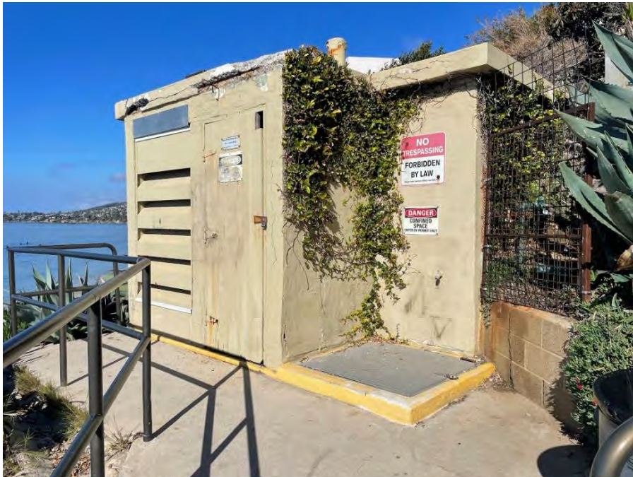
Photo 6: View of the lift station in the middle portion of the staircase. Viewing north.
