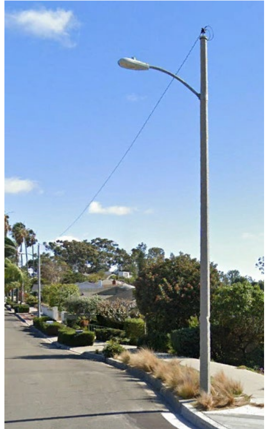
Alta Laguna Blvd. at Temple Hills Drive (overhead wiring)
