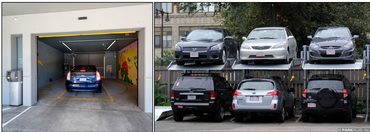
Figure 29 and 30. Left: The City of West Hollywood City Hall has an automated garage system. The mechanical system stores and retrieves vehicles. Photo credit: City of West Hollywood. Right: Double-stack mechanical lift. Photo credit: Park Plus, Inc.
