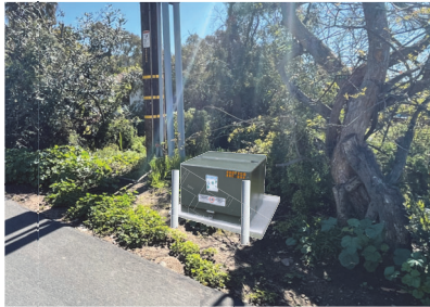
SDGE PAD-MOUNTED TRANSFORMER 36" x 33" x 26" (DARK GREEN FINISH) W/ TWO BOLLARDS
