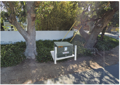
SDGE PAD-MOUNTED TRANSFORMER 36" x 33" X 26" (DARK GREEN FINISH)
