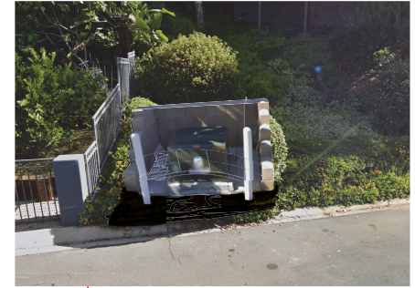
SDGE PAD-MOUNTED TRANSFORMER 36" x 33" X 26" (DARK GREEN FINISH) W/ TWO BOLLARDS & CONCRETE MASONRY RETAINING WALL (SANDSTONE COLOR)
