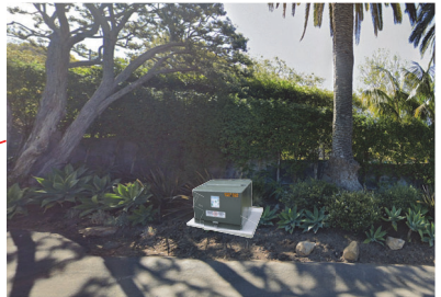
SDGE PAD-MOUNTED TRANSFORMER 36" x 33" x 26" (DARK GREEN FINISH)
