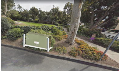
SDGE TERMINATOR CABINET 68" x 22" x 33" (DARK GREEN FINISH) W/ TWO BOLLARDS
