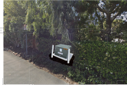
SDGE PAD-MOUNTED TRANSFORMER 36" x 33" x 26" (DARK GREEN FINISH) W/ TWO BOLLARDS
