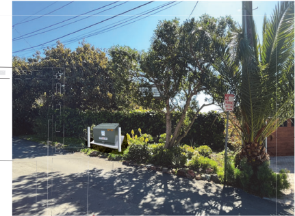
SDGE PAD-MOUNTED TRANSFORMER 36" x 33" x 26" (DARK GREEN FINISH) W/ TWO BOLLARDS
