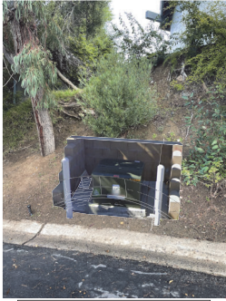
SDGE PAD-MOUNTED TRANSFORMER 36" x 33" X 26" (DARK GREEN FINISH) W/ TWO BOLLARDS & CONCRETE MASONRY RETAINING WALL (SANDSTONE COLOR)
