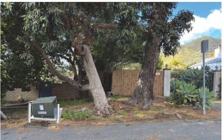
SDGE PAD-MOUNTED TRANSFORMER 36" x 33" X 26" (DARK GREEN FINISH) W/ TWO BOLLARDS
