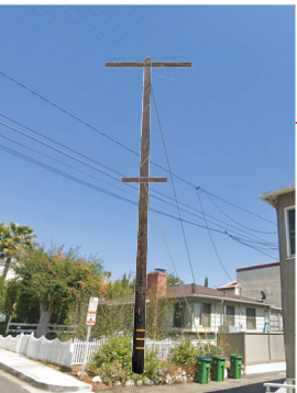
NEW INTERSET UTILITY POLE 55" HEIGHT w/ DOWN GUYS
