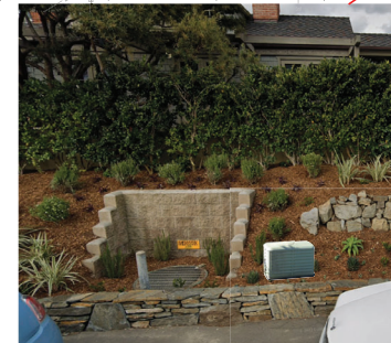
NEW COX LOWBOY PEDESTAL TO REPLACE EXISTING PEDESTAL 24" x 36" x 21" LIGHT GREEN COLOR (AFTER)
