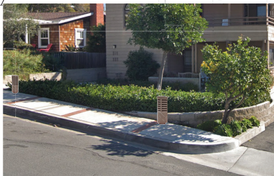
SCE VENT STANDPIPES 10" DIAMETER, 34" HEIGHT SANDSTONE (BROWN) FINISH
