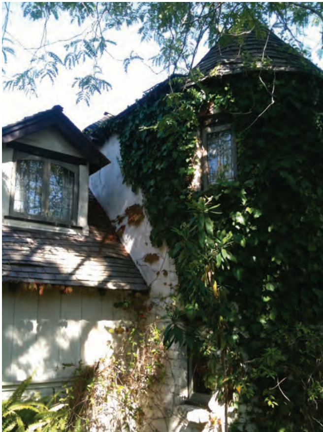
This home at 820 Catalina Street was built in the eclectic Tudor style around 1929. The home is in good condition and maintains a E rating on the city’s historic register.
